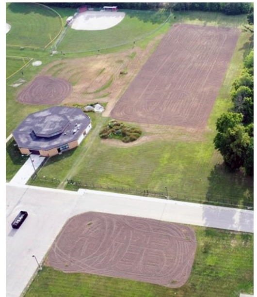
Phase One of the BCAP project is underway with the construction of athletic and baseball fields, a pickleball court and additional parking.
